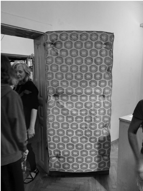
The sound proofing mattress door.
