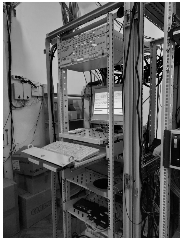
The central control unit of the server rack.
